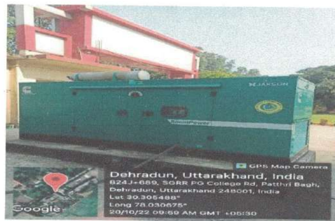
Fig-34: 82.5 KVA DG Set installed in SGRR University, Pathribagh
