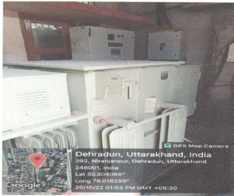
Figure-3.2: 11/0.4 KV Sub Station of ITS SGRR University
